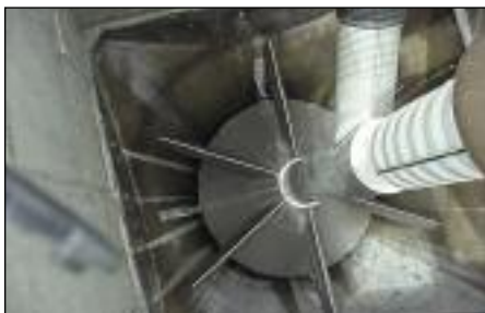
DynaSand Filter modules in concrete basin
