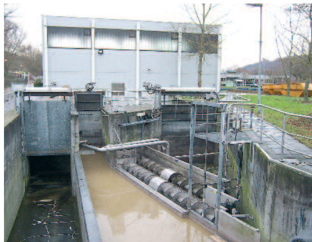
Combination of different screening systems for optimised treatment of large volumes of wastewater
