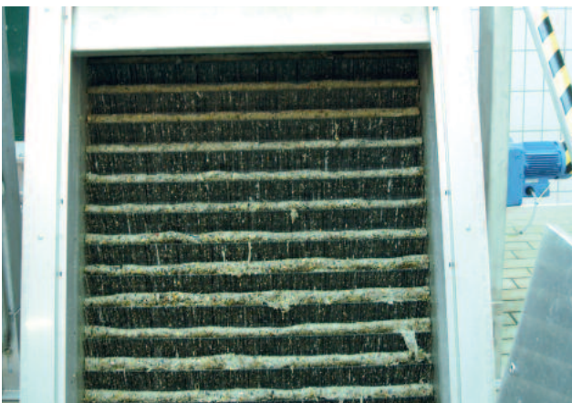
STEP SCREEN® Vertical SSV: very high separation capacity due to the fine slot widths and the produced screenings carpet
