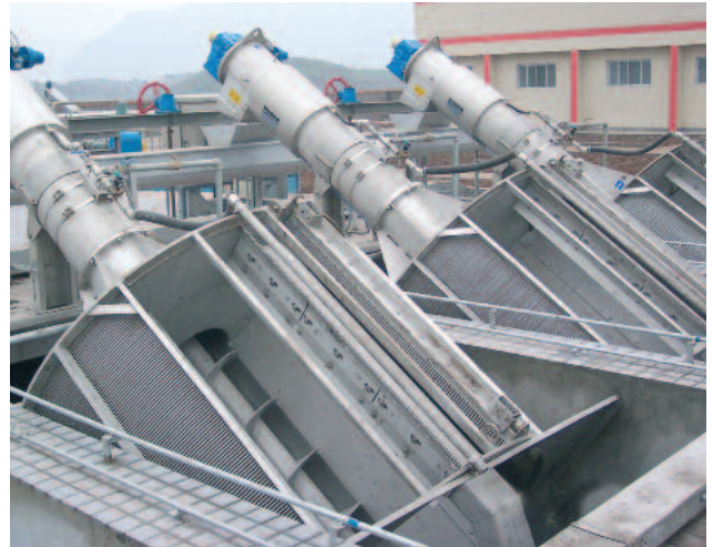
Several parallel ROTAMAT® Fine Screens installed in the channel
