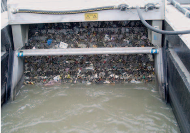
STEP SCREEN® Flexible SSF: length 3500 mm, width 1826 mm, 6 mm slot width, 50° installation angle. High capacity as the flow passes the screen surface only once.
