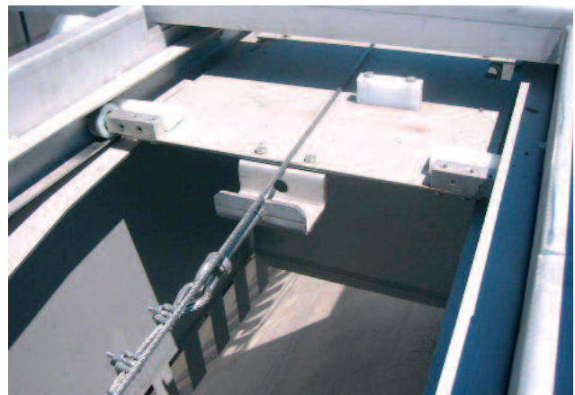
Semi-automatic grease removal by means of a paddle system
