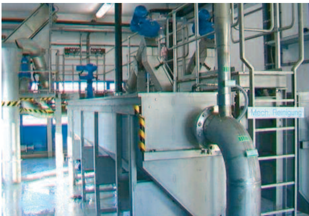
Above-ground redundant installation of Grit Trap Ro6
