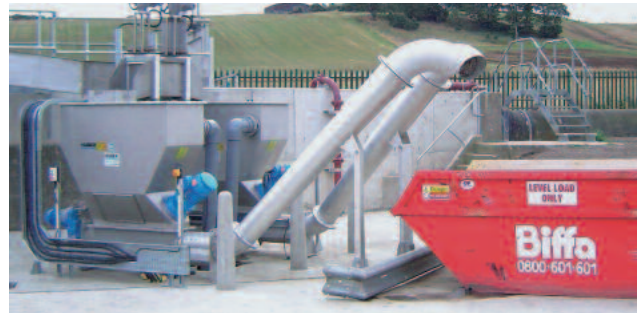
Outdoor installation of a HUBER Screenings Wash Press WAP/SL
