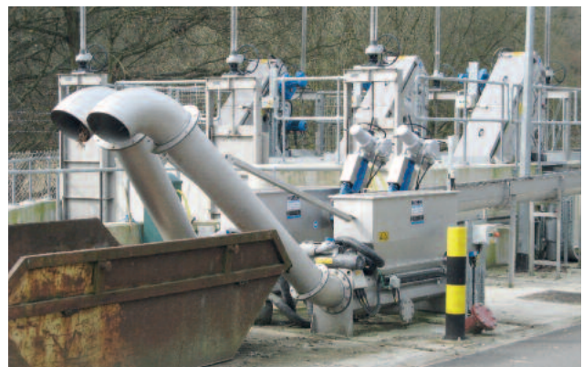
Redundant operation and optimal screenings dewatering with launder channel feeding system
